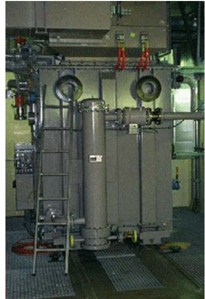
Installed ABB substation power transformer rated 5 MVA.
